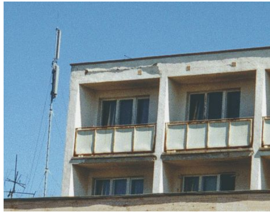
Figure 2: A horizontal crack formed on the facade wall
