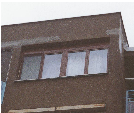
Figure 4: Wrongly repaired horizontal crack on facade wall
